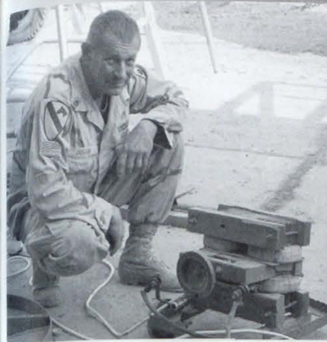
Bravo Company fabricated all armor for vehicles throughout the Brigade while manufactured armor was unavailable. The company also installed Red Dot air conditioning units on armored vehicles and gained the reputation as the most productive maintenance unit in Theatre with over 4500 hours of labor logged in support of the 39 th Brigade.
